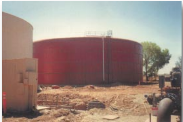
Construction of a two-million-gallon reservoir was one of the short-term improvements designed and implemented by Brown and Caldwell for the Cordova System.
